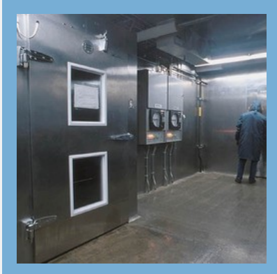
Cold Storage Equipment
